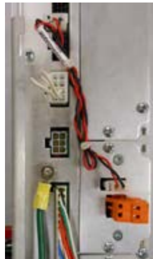
Figure 7-12. DC power supply (13.5 Vdc) installed in the side of a CL-7 control.
