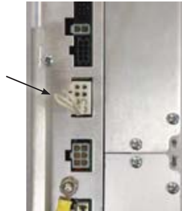
Figure 7-11. DC power jumper in place on side of control. This jumper must be in place to power the control when the substation battery option is not provided.
